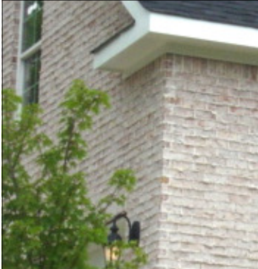
Brick with Weeping Mortar
