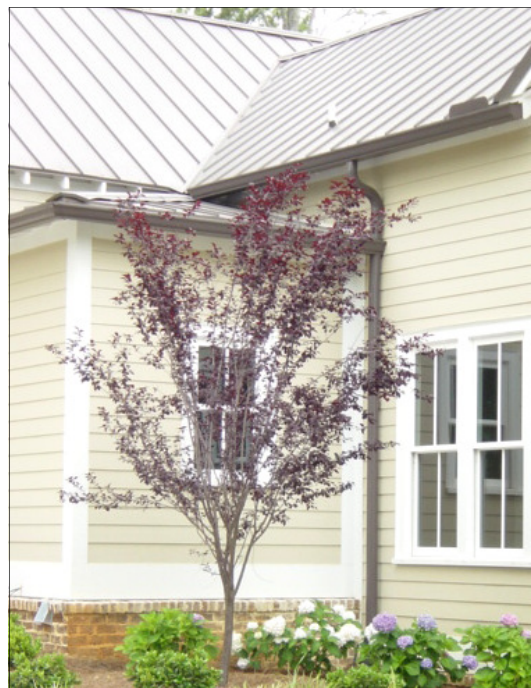
Hand-Crimped Standing Seam Roof
