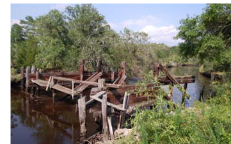
Remains of a dam gate used to maintain desired water levels
