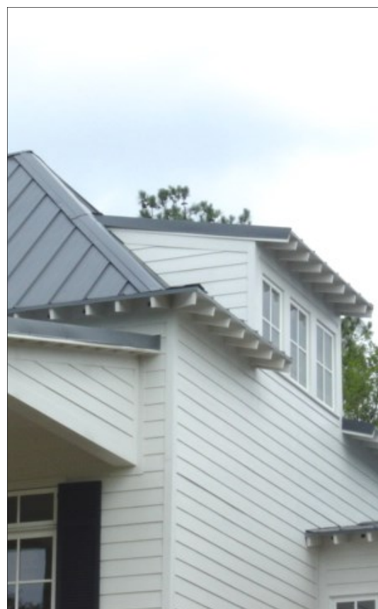
Exposed Rafter Tails
