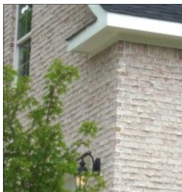
Brick with Weeping Mortar
