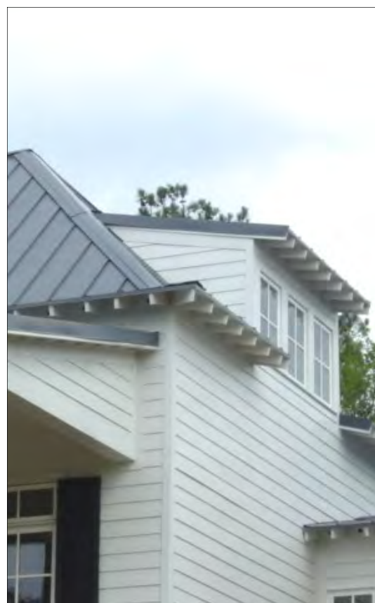
Exposed Rafter Tails
