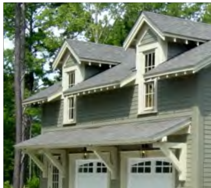
Exposed Rafter Tails
