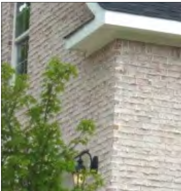
Brick with Weeping Mortar
